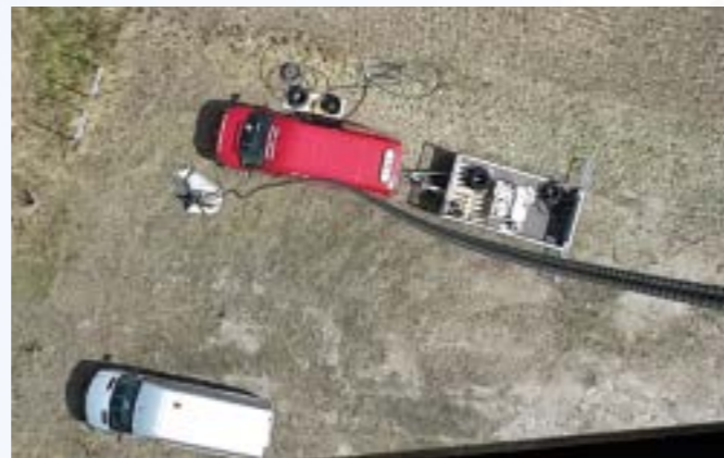
» All maintenance and repair operations involve a great deal of careful planning. Two service technicians have to carry the necessary materials and tools more than 90 m up into the air by means of a crane.
